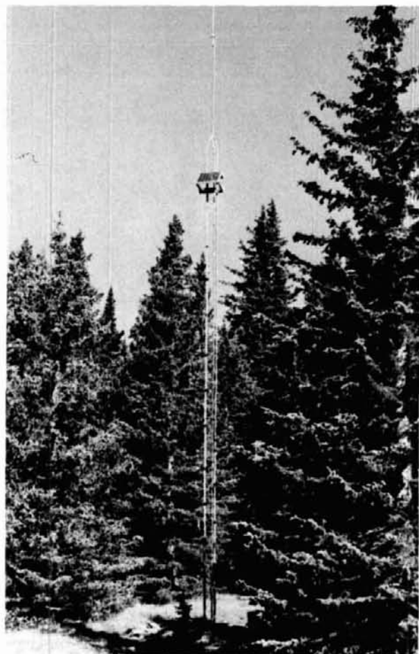
Redondo Peak repeater installation. Solar array is mounted near the top of the tower to prevent shading. The repeater electronics are installed underground at the base of the tower.
